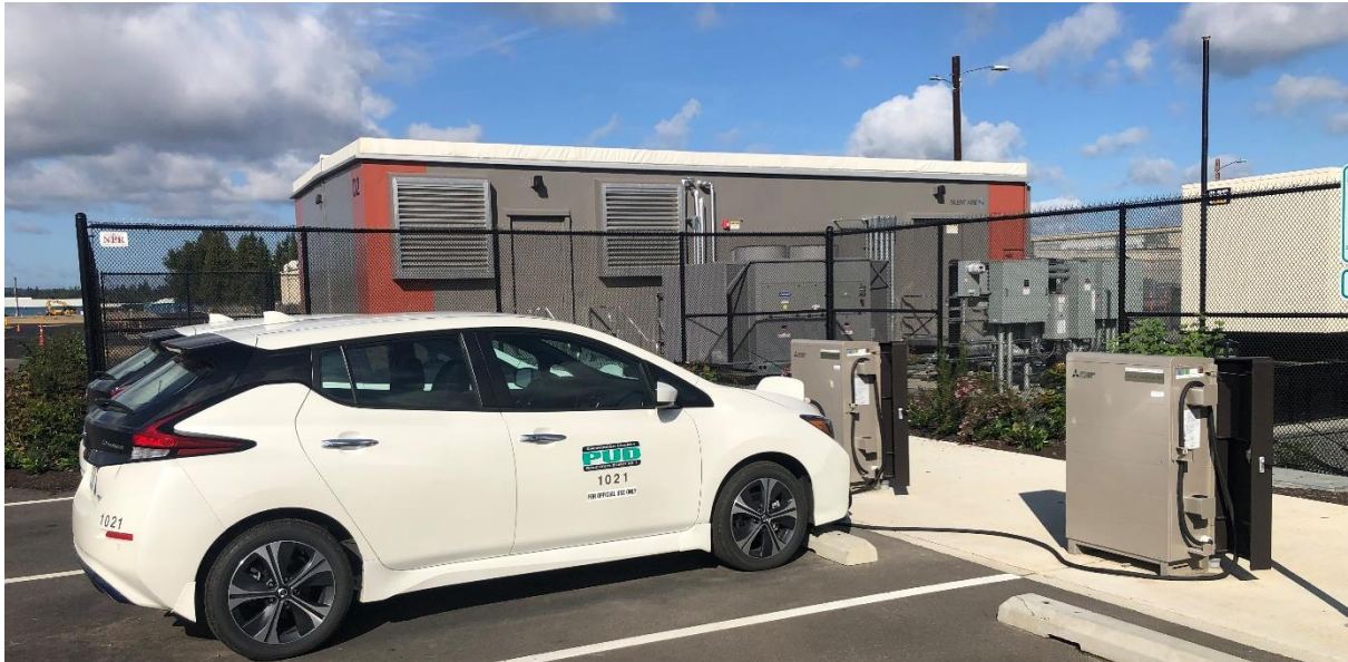
Figure 3 : These light-duty electric vehicles charge and discharge power into the Arlington microgrid and PUD grid
